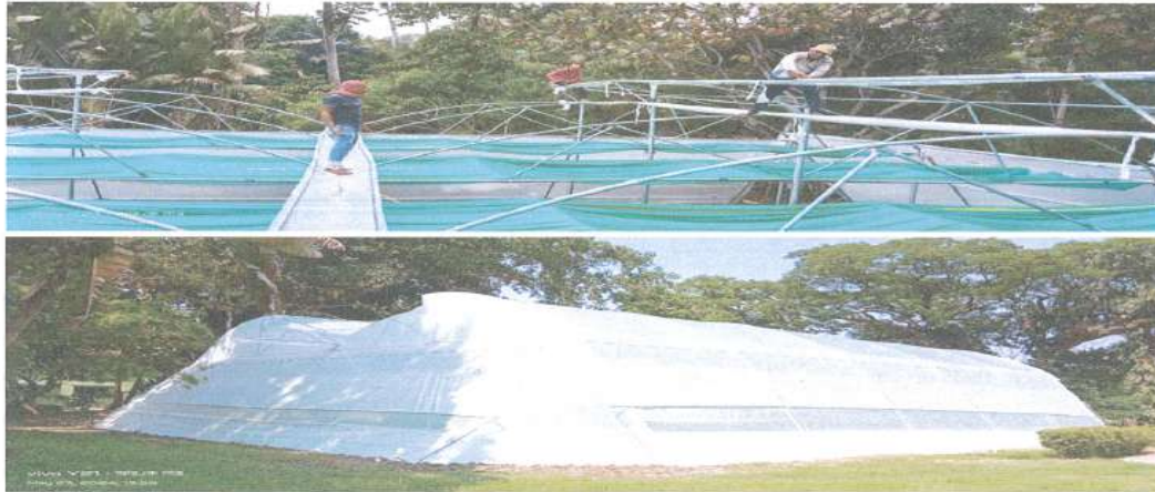
Different stage of development of construction of the Naturally ventilated poly house
