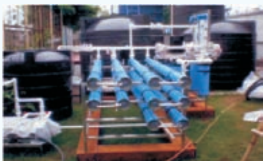
Tertiary Level Treatment by provision of Reverse Osmosis (Source-SPCB)
