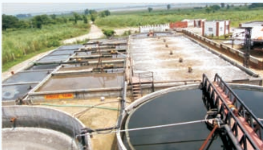
Effluent Treatment System for Treatment of Industrial Waste Water
