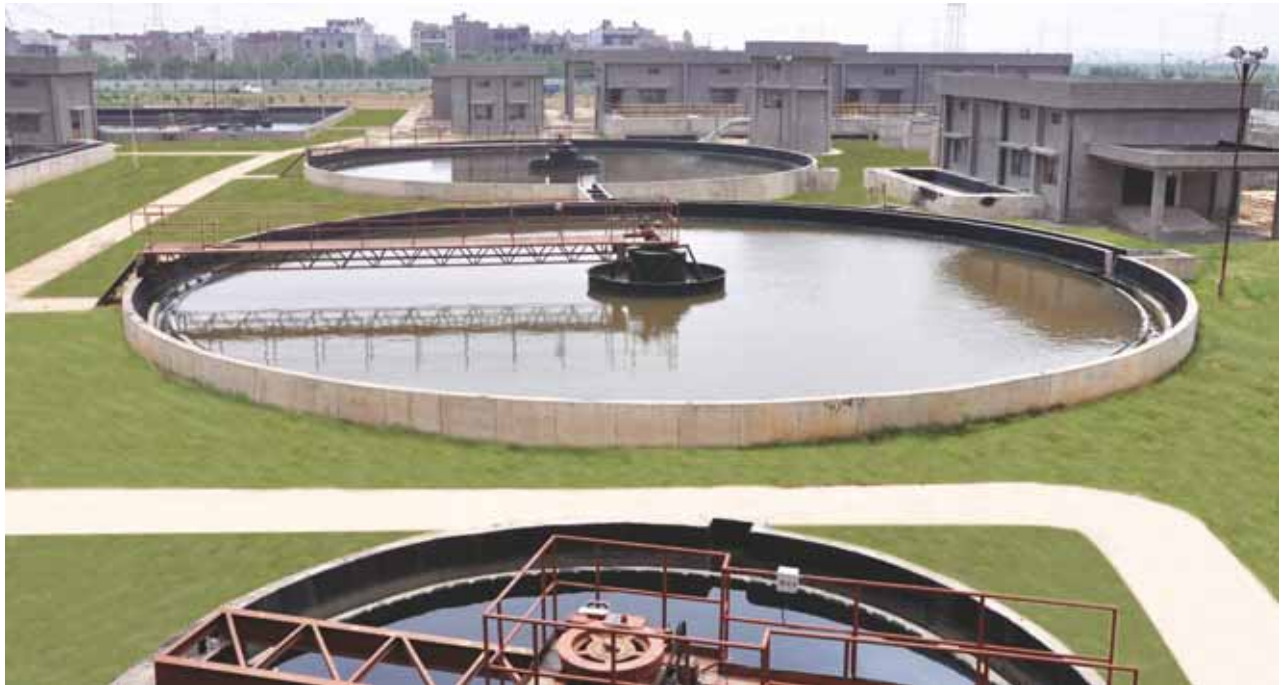
Fig. 32 35 MLD Bawana Common Effluent Treatment Plant in Delhi
