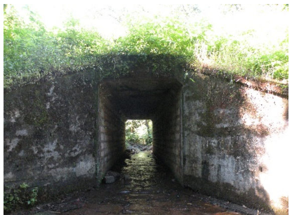
Effectiveness of existing underpasses such as this one below Dudhsagar railway track should be evaluated (Photo: A. J. T. Johnsingh)
