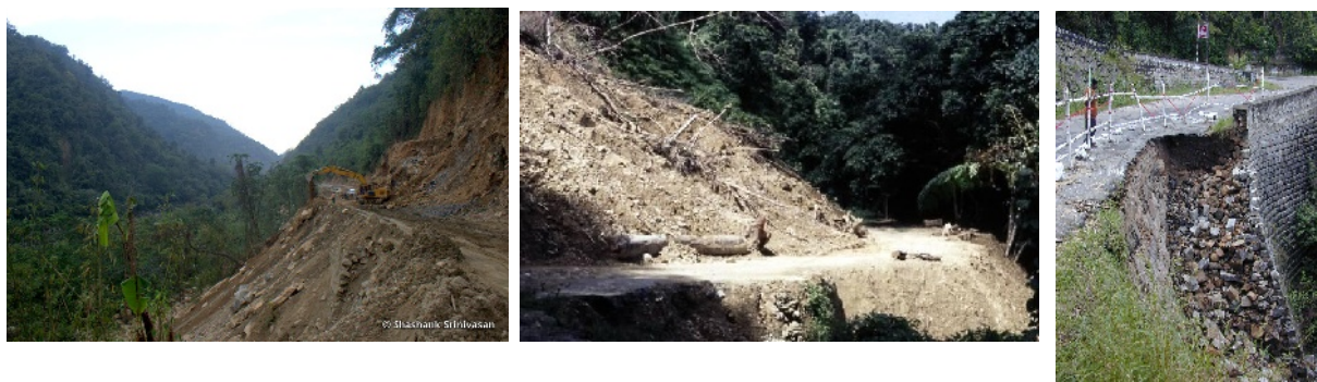
From left to right: Widening and earth dumping on road to Tawang near Pakke Tiger Reserve (Photo: Shashank Srinivasan); landslide on E-W Road in Great Nicobars (Photo: Manish Chandi); hard engineering methods are poor replacement for natural vegetation to prevent erosion and slips (Photo: NCF)
