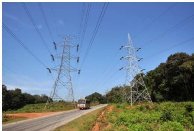
Transmission lines double up with a road through forests in Karnataka (Photo: NCF)
