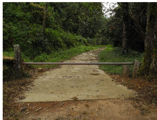
A section of road concrete-topped through montane shola in Anamalai Tiger Reserve (Photo: NCF)
