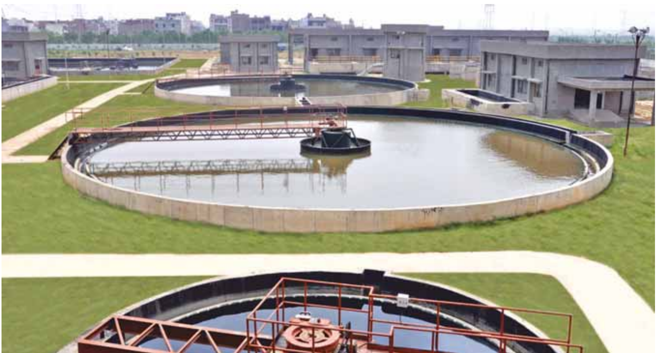
Photo 9.5: Waste water treatment plant
