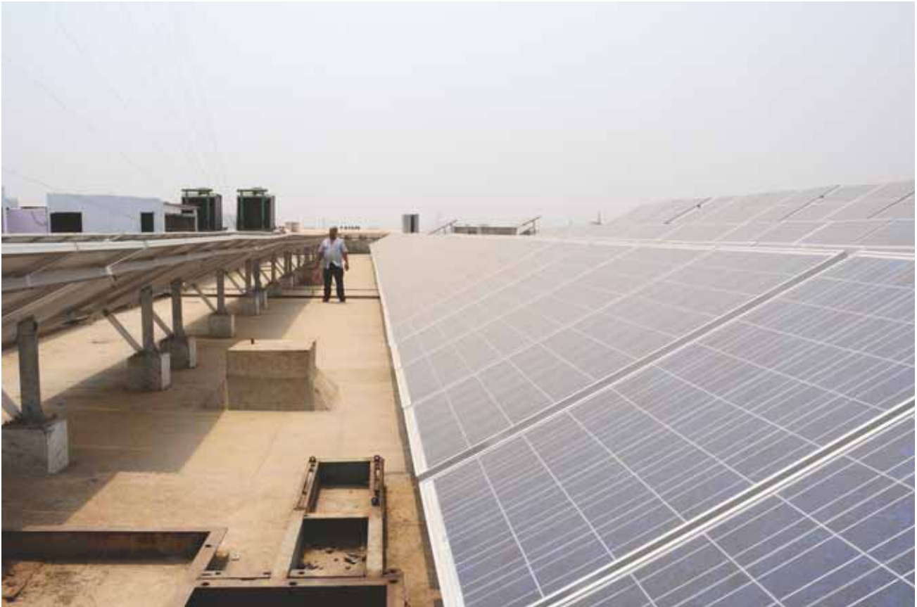
Photo 6.3: Roof top solar panels
